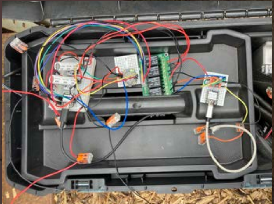
<Experimental setup for powering the XIAO with two Li-ion capacitors with a power switching system>
